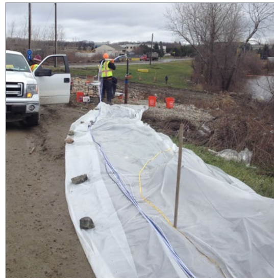
Five Waterloo Systems were installed to 33.5 m (110 ft) in fractured bedrock to help characterize a historical chlorobenzene plume at the site of a proposed groundwater pump and treat site. Vibrating Wire Transducers and Double Valve Pumps were dedicated at each of the 4 monitoring zones.
